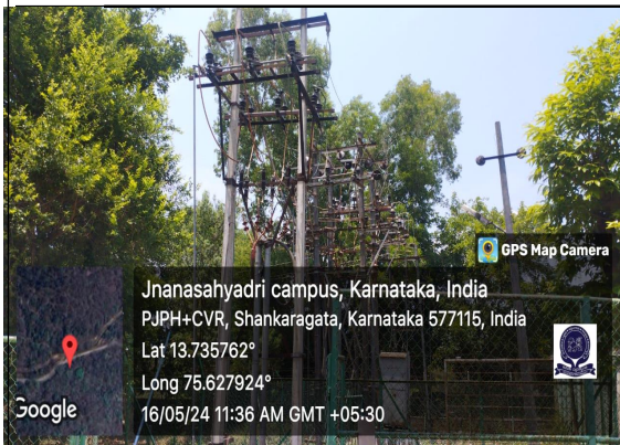
Power transformer unit 1
