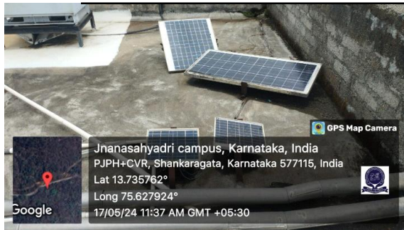
nergy units installed on campus buildings
