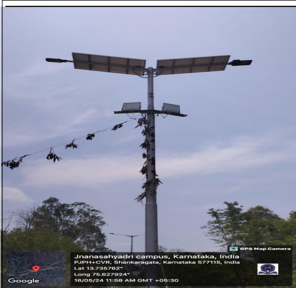
Solar Street light with LED bulbs
